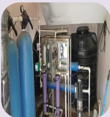
R.O. WATER PLANT
